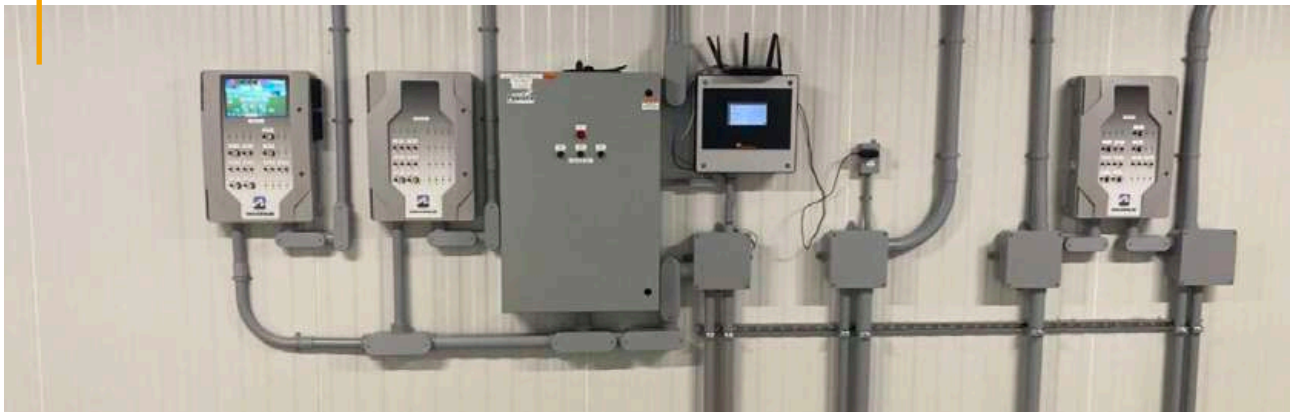
Ventilation controllers from a local supplier that are made in Canada are used in this new barn.
